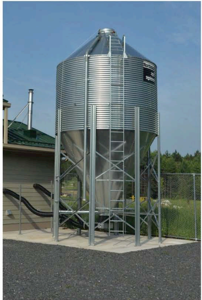
Wood pellets are bulk-delivered to the facility and blown into an outdoor hopper, from which the boilers automatically draw when needed.
