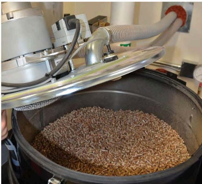
The wood pellets that fuel the boilers are sawmilling byproducts. Only compressed wood is used in the making of the pellets, no bonding agent. They're seen here inside one of the boiler's "day bins."
