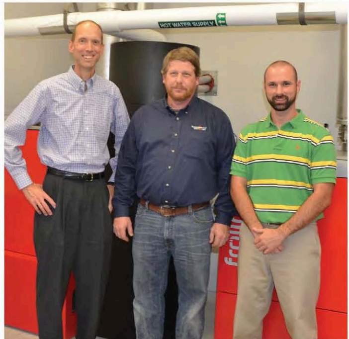
(L-R) Carl Longenecker, owner of ATI Systems, René Ferland, sales & technical support for Tarm USA, and Jason Adams, C.B.C.P Mechanical Engineer II, with Pennsylvania DCNR, stand in front of the two pellet boilers.
